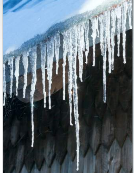
RX Roof & Gutter De-Icing
